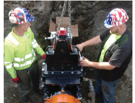
The crew completed the project over the course of 2 days without shutting down the line.
