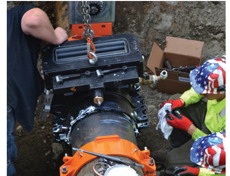
The installation team places the valve body to begin the installation on the 100-year old cast iron pipe.
