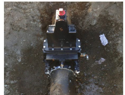
The first project using an AVT EZ Valve designed for a 14-inch (350-mm) line was executed according to plan, delivering a perfect installation.
