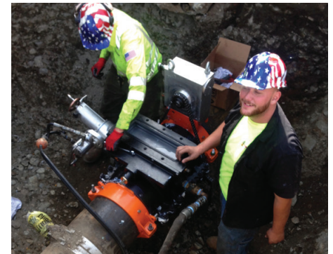
Installers prepare to make a cut in the line using the AVT EZ Valve, newly designed for a 14-inch (350-mm) line.
