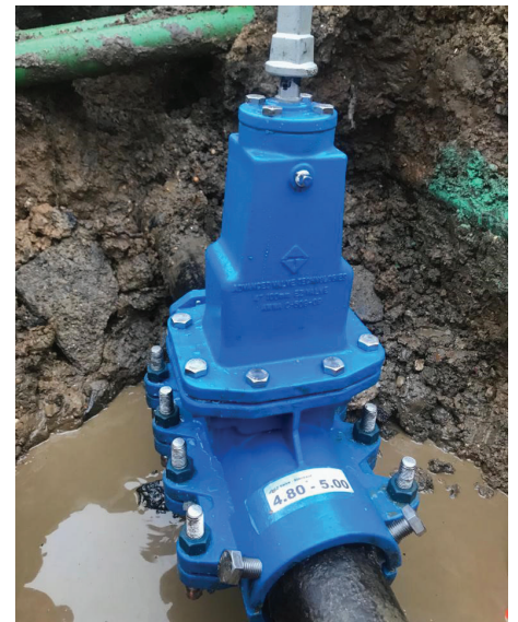
Two technicians installed the 4-inch (100-mm) AVT EZ Valve on a cast iron potable water pipeline in two hours, delivering a durable solution without interrupting service. (Photo courtesy of R2M Ltd.)
