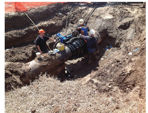
The first of three 24-inch (600-mm) EZ Valves is installed to control the main feed pipes in Ponca City, Oklahoma.
