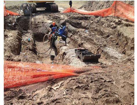
24-inch (600-mm) AVT EZ Valves were installed on three ductile iron pipe municipal water mains.
