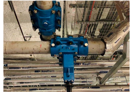
10" AVT EZ Valves fitted to horizontal and vertical LTHW lines in a UK hospital
