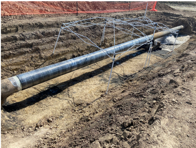
Figure 1. Atlas has been used to permanently reinforce crack-like defects on this 16 in. pipeline.
