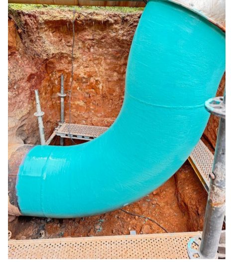
EPN 242 putty was applied to smooth the surface, followed by PPR 290 as a corrosion inhibitor.
