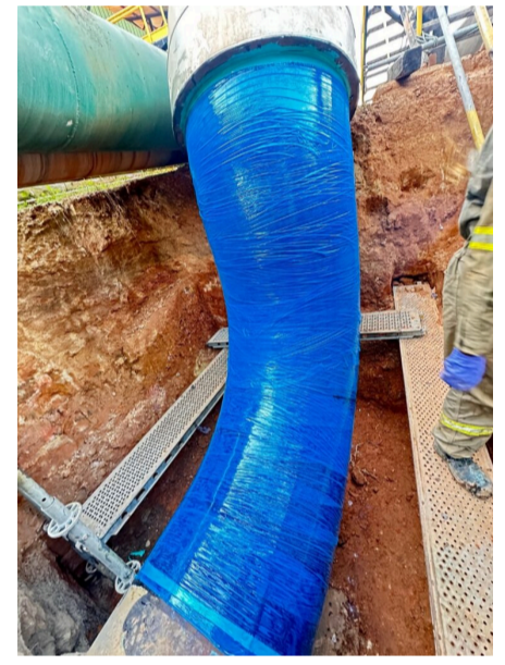
Compression film is applied to the repair to accommodate the release of excess resin.
