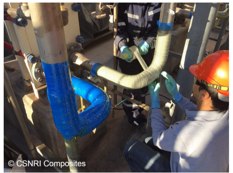
AcidShield restored the damaged stainless steel pipe to original design strength without interruption of operation.
