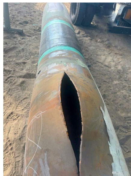
The repair was tested to 2800 psi, resulting in a failure to the pipe body, but not to the Atlas repair, which was designed for 1200psi.
