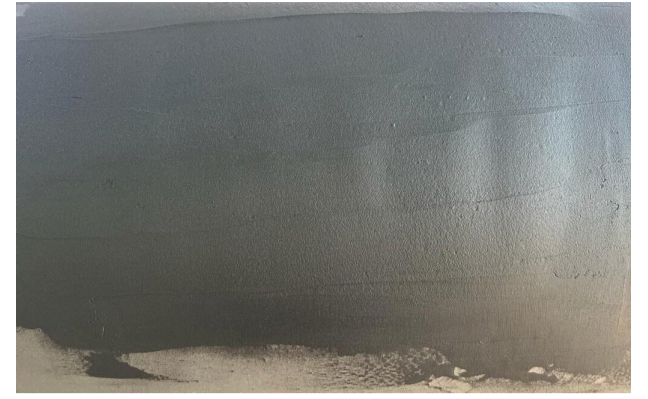
The pipe geometry was smoothed with EPN 242 putty prior to the application of the Atlas wrap.
