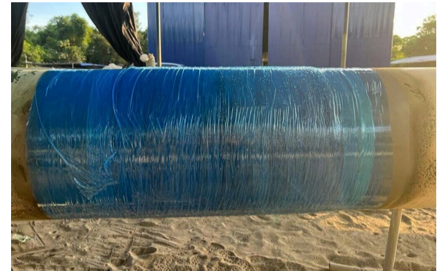
Compression film was applied over the repair and perforated, then allowed to cure.
