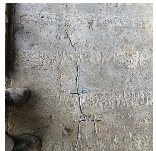
Cracked and spalling concrete
