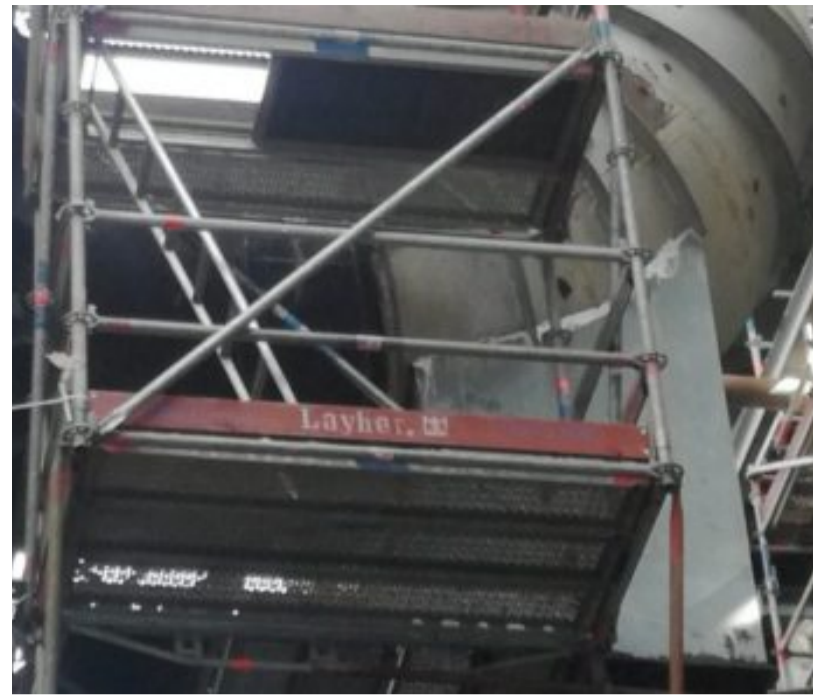
Because of the location of the line, special scaffolding was built to give technicians access so they could wrap 508-mm (20-inch) wide swathes of fiber carbon cloth around the 2,000-mm (78.7-inch) diameter flare line.
