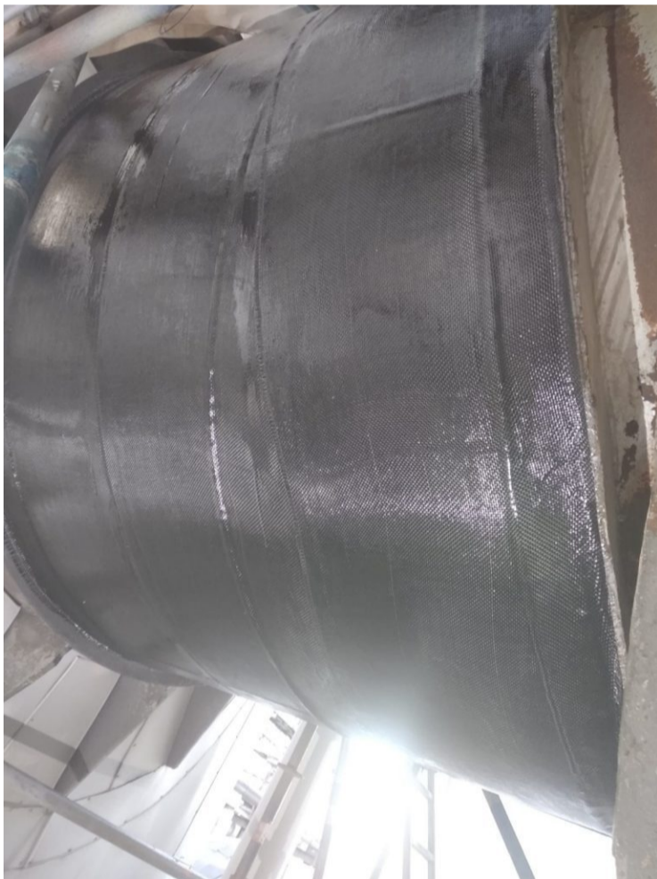
Installers completed the repair within 4 working days of the initial inquiry without introducing negative environmental risks or hot work and without disrupting refinery operations, providing a solution that delivers an additional 2 years of safe service.
