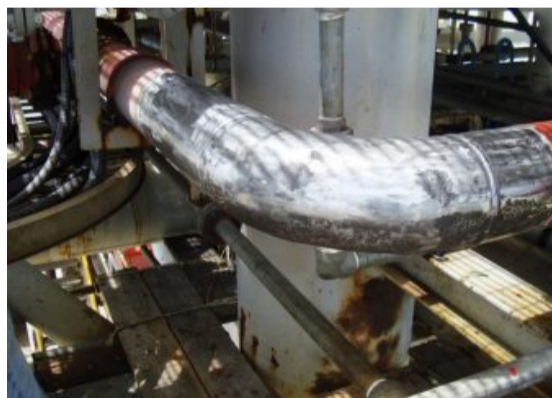
Installers used power tools to clean the spool sections in preparation for the composite repair.
