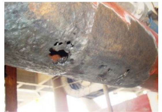
Corrosion led to multiple through-wall defects on an 203-mm (8-in) diameter firewater line on an offshore platform.
