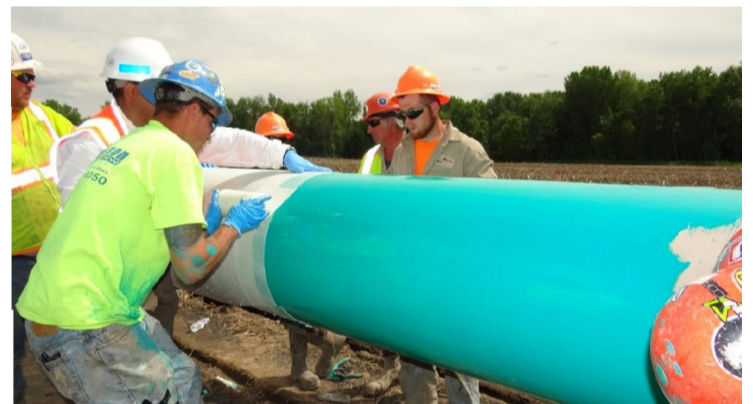
The installation team prepares a 300-ft (91-m) section of pipe with ScarGuard for a test pull.
