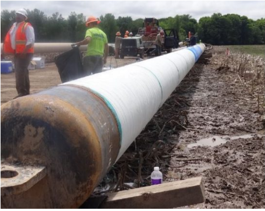
The field team wrapped 300 ft (91-m) of the line and every weld with ScarGuard to provide maximum protection during the installation, enabling the successful HDD installation of the full 1,200 feet (366 m) of pipe.
