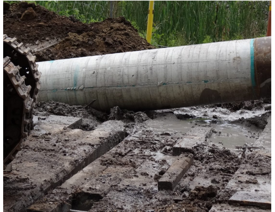
A successful test pull proves that ScarGuard is equal to the task of protecting the pipe from abrasion from the cobble.
