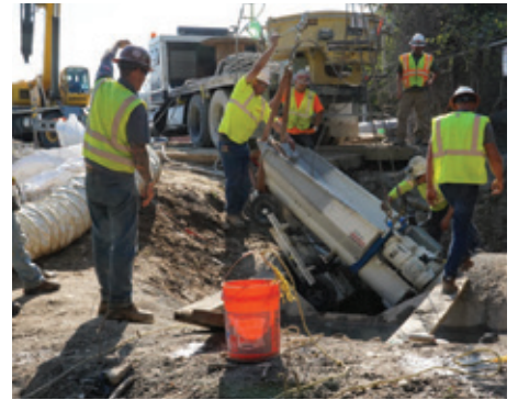
All work was done from a single entrance point at the project site
