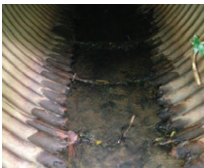
Initial pipe conditions were extremely poor.
