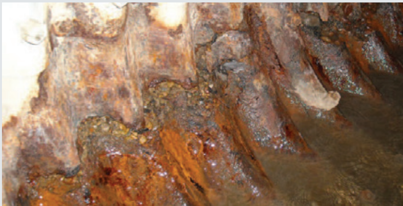
Corrosion along water line with rusted through sections.
